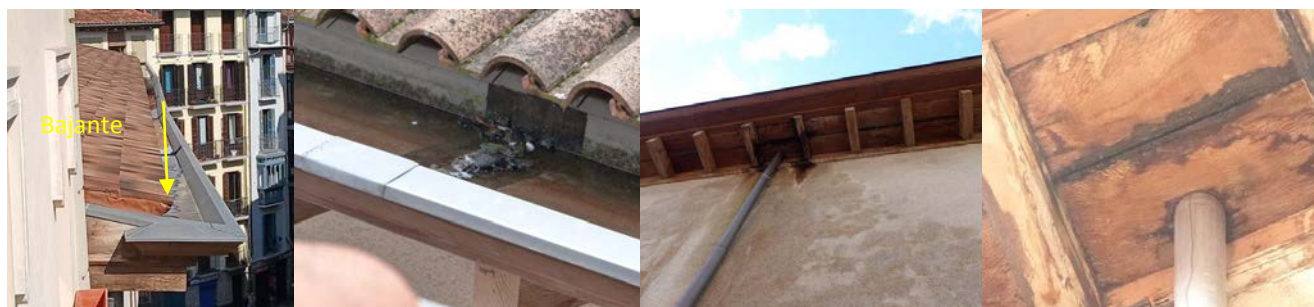
Bajante canalón C/ Mayor
