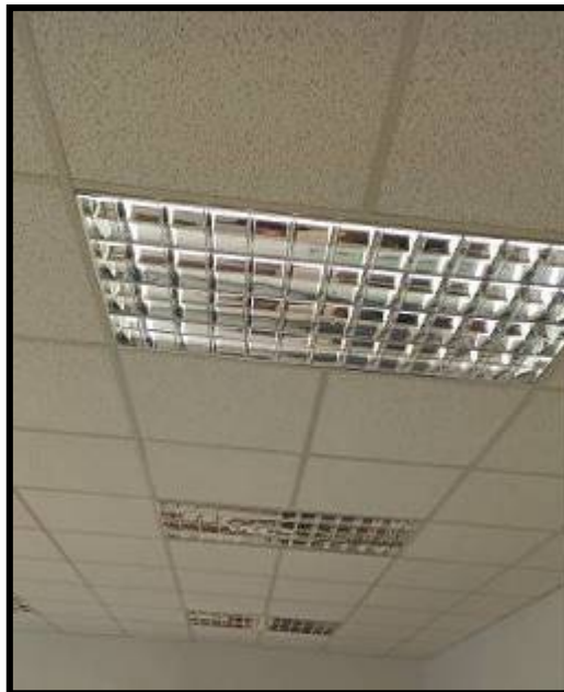
Luminarias fluorescentes 4x36 W.
